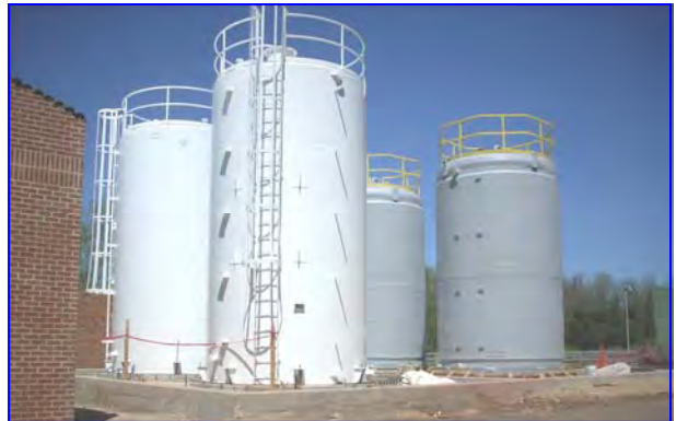
New Bulk Chemical Storage
