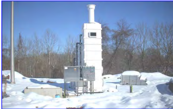
New Chemical Scrubbers for Odor Control
