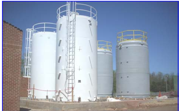
New Bulk Chemical Storage
