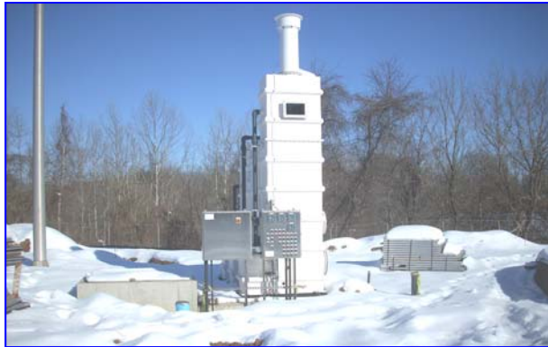
New Chemical Scrubbers for Odor Control
