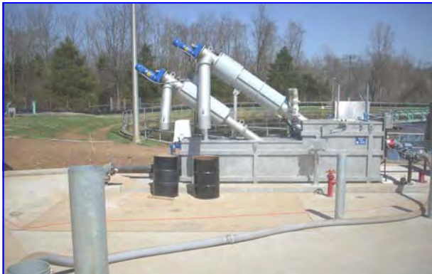
New Septage Receiving Station
