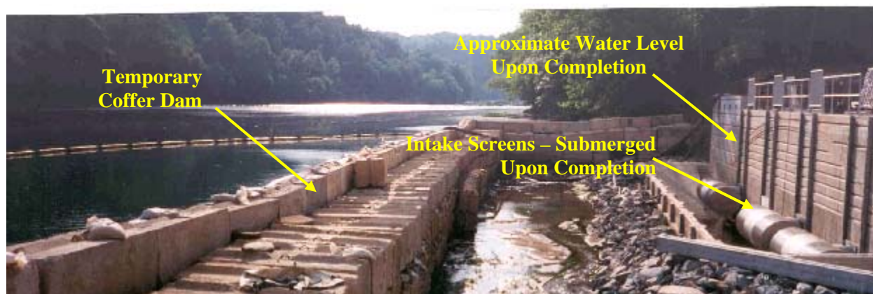
Figure 3: Side River Intake Structure Under Construction (Pump Station Off Picture to Right)
