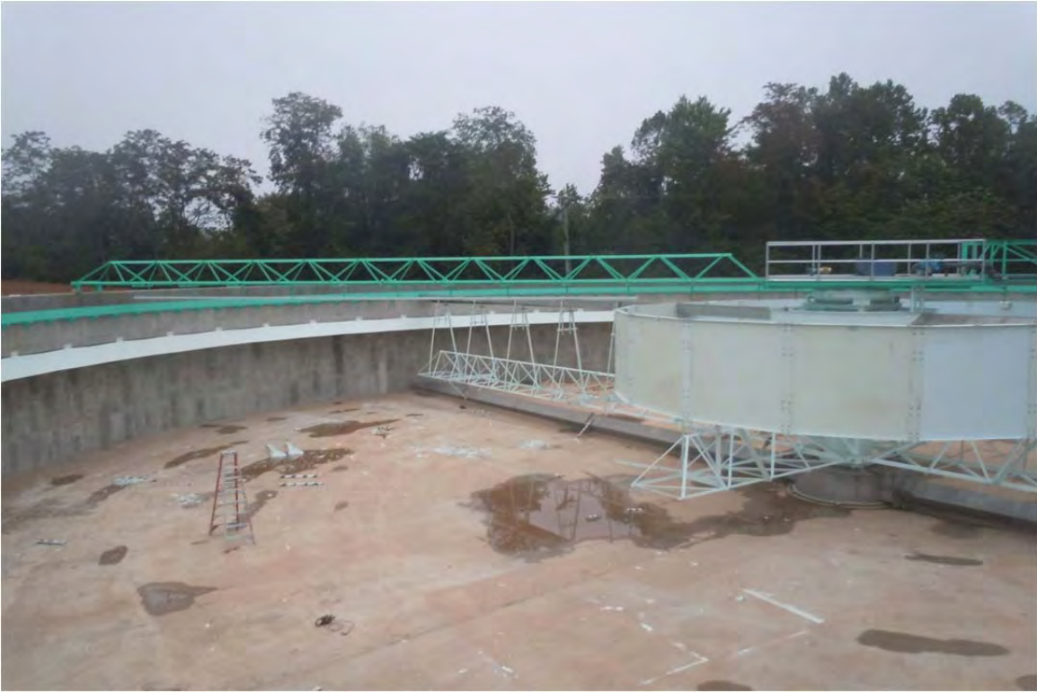
New Secondary Clarifier Mechanism
