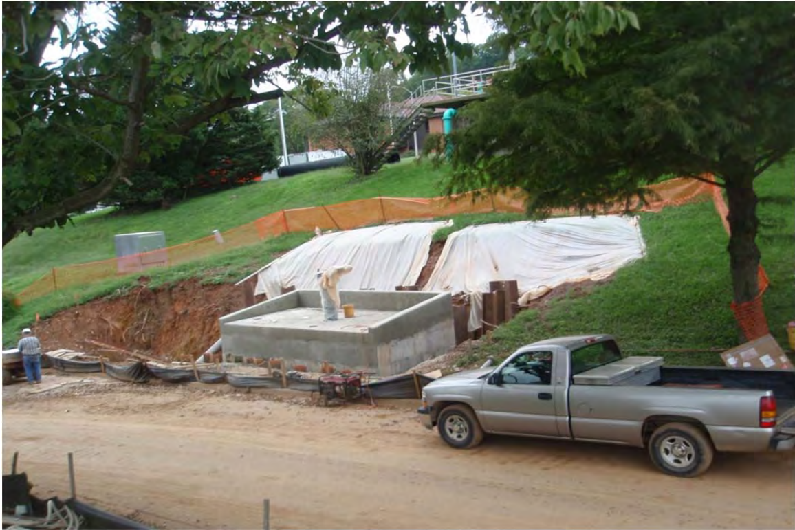
Holding Pond Force Main Metering Vault
