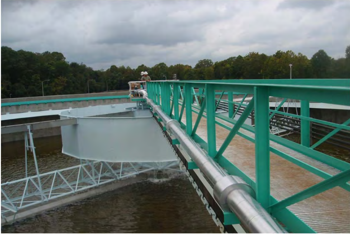
Catwalk and Centerwell of Secondary Clarifier No. 4
