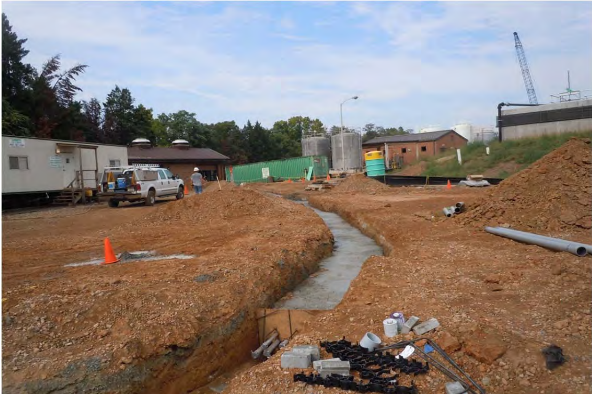
Electrical Duct Bank to Secondary Clarifier No. 4
