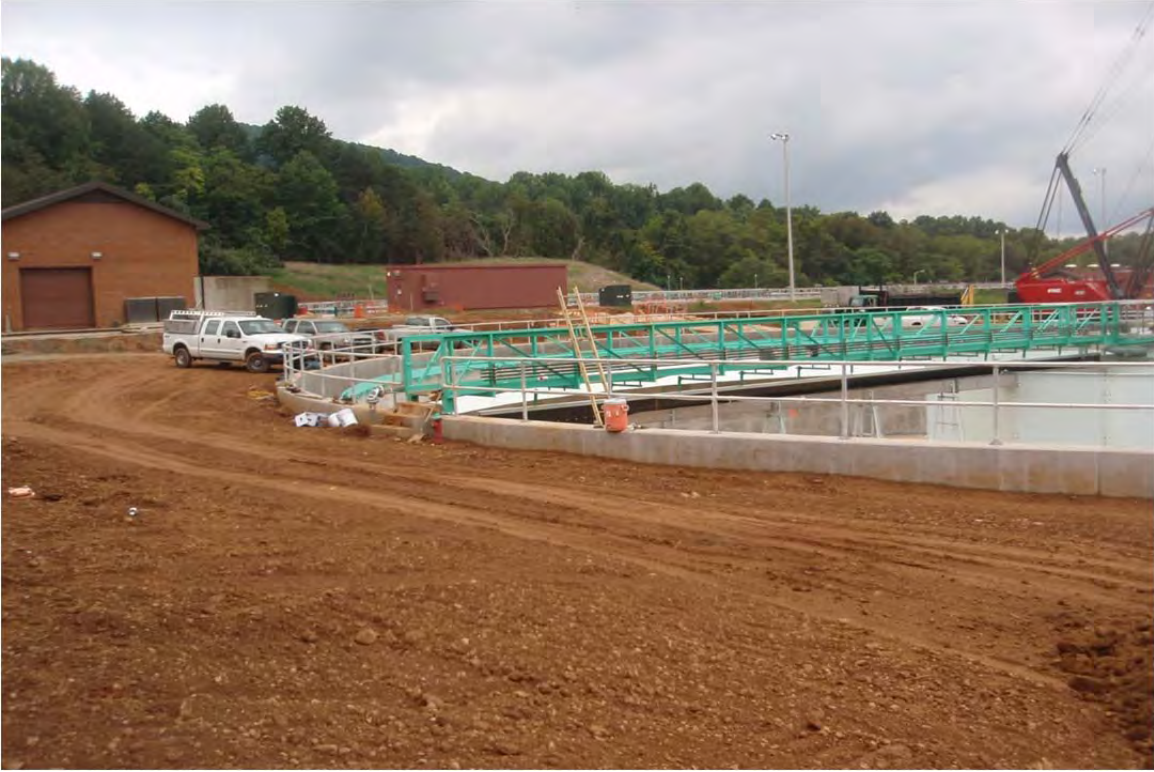
Secondary Clarifier No. 3
