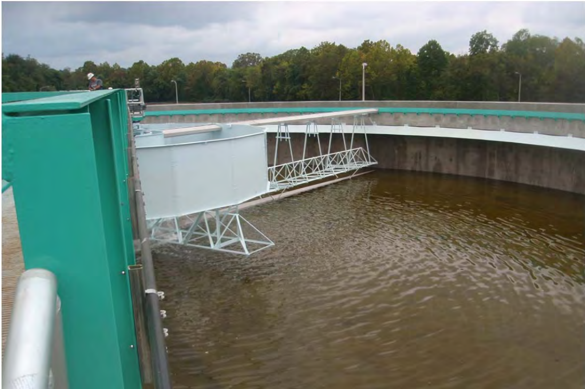
Secondary Clarifier No. 4
