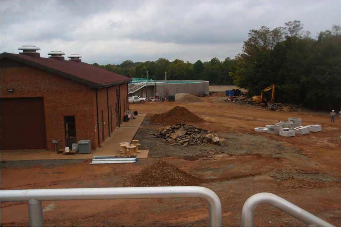
View from Aeration Basins in the Maintenance Yard with Secondary Clarifier No. 4 in the Background
