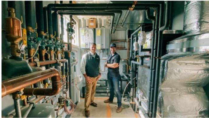
Energy Efficient Mechanical System
