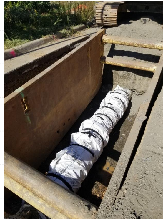
Airport Road Pump Station Line
