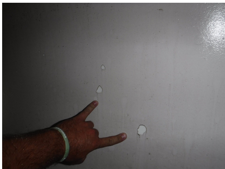
24) Minor topcoat delamination on the sidewall.
