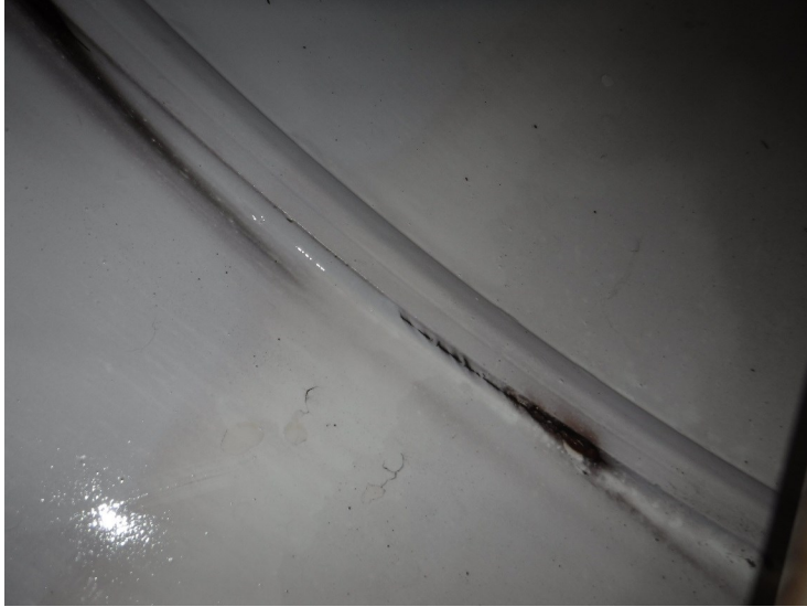
28) The roof coating is in good condition with minor cracking of coating at the weld seams.
