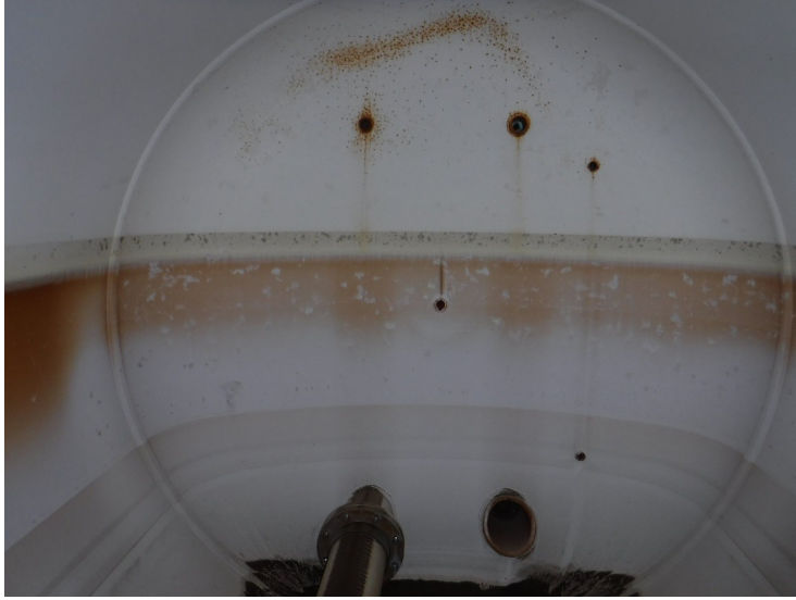
34) Coating on endcap is in good condition with minor rust bleedthrough.
