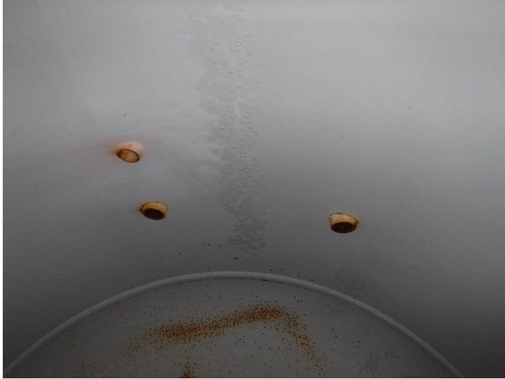
25) The roof coating is in good condition overall with coating failures on roof couplings.
