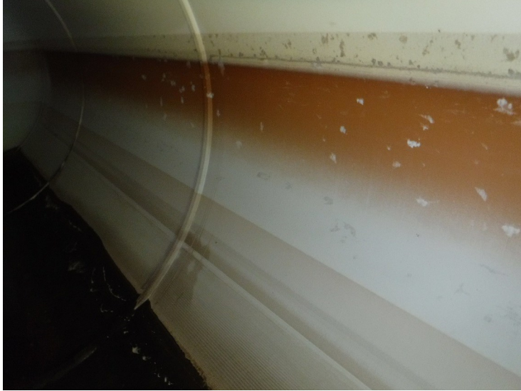
22) The sidewall coating is in good condition with mineral staining at the equator.
