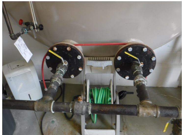
17) Piping inside of building is not coated and has some minor surface rust.
