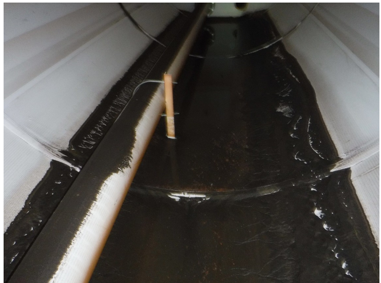
20) Bottom of tank was covered with sediment.
