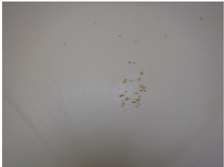
26) Minor rust bleedthrough on the roof.
