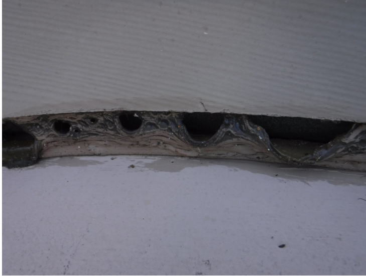
16) Caulking between the building and the tank is missing on the top.
