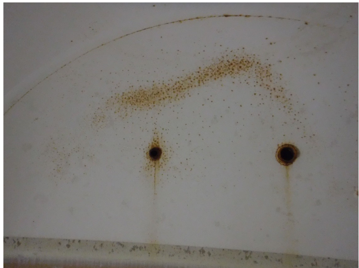
35) View of rust bleedthrough and couplings in the end cap.
