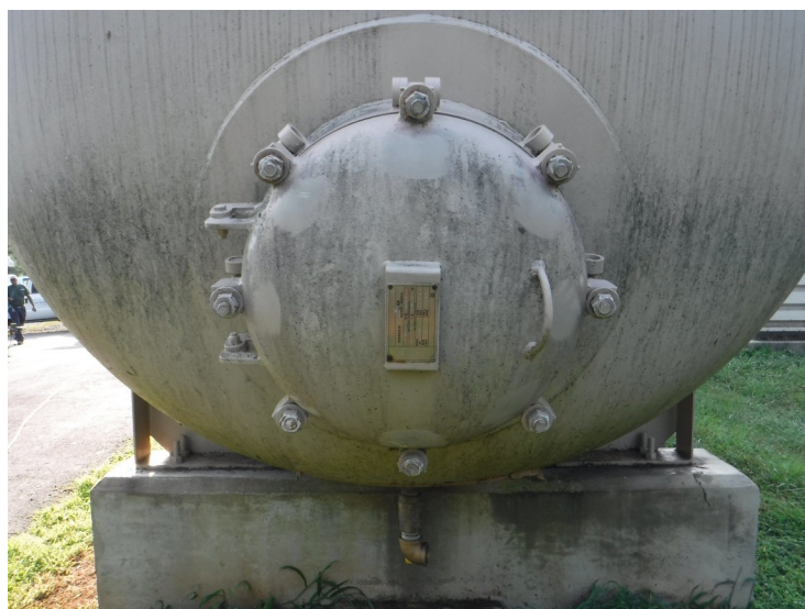
15) Manway to wet interior on exterior endcap.
