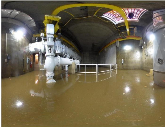
Submerged pump station pump room
