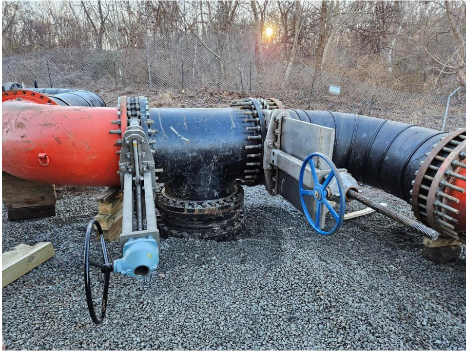
Bypass system pipes
