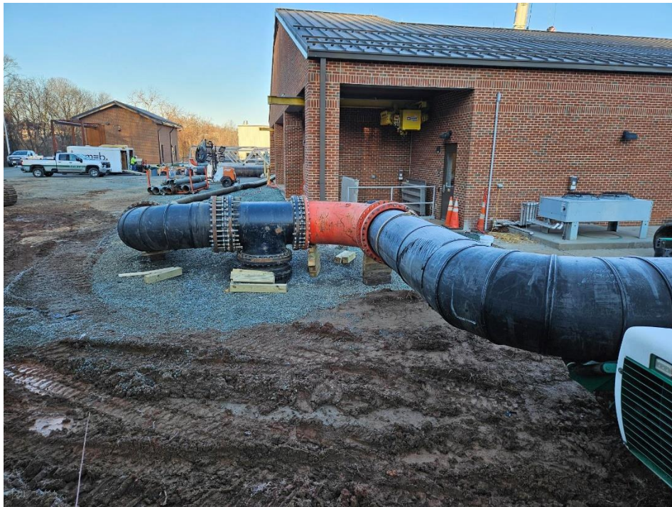
Bypass system pipes
