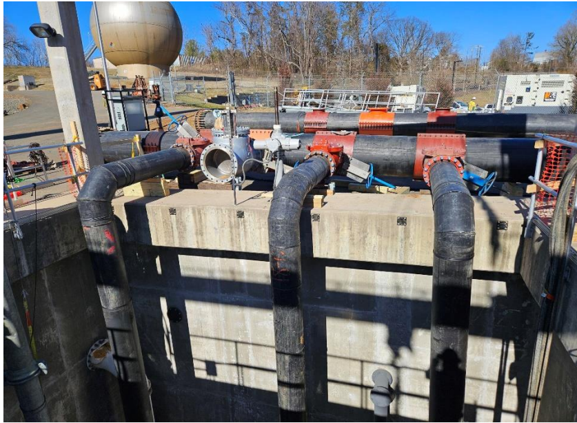
50 million gallon per day bypass
