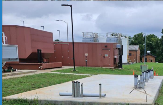
Concrete Pad for Motor Control Center
