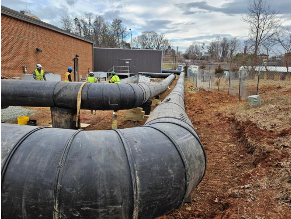
Large bypass system pipes
