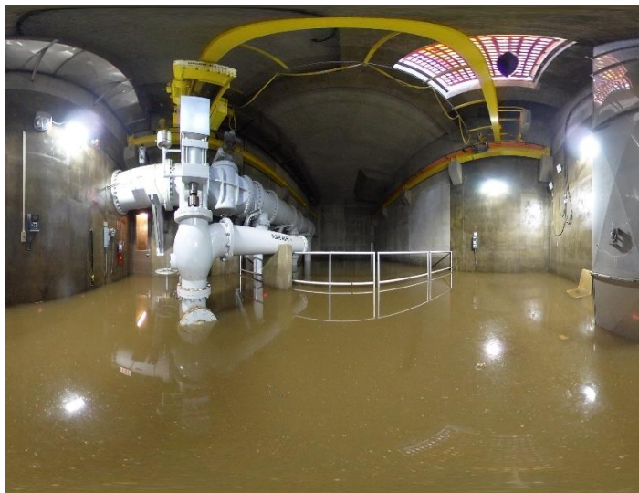
Submerged pump station pump room
