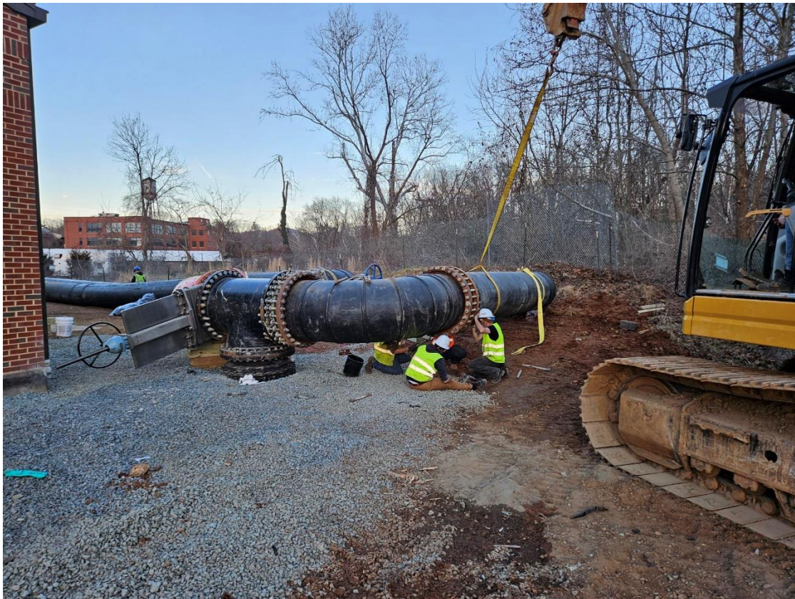
Bypass system pipes
