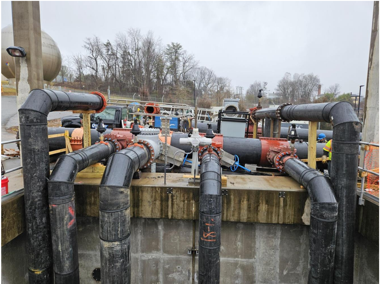
Bypass pumping system
