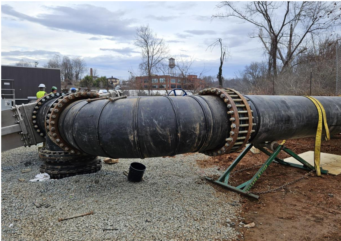
Pumping bypass system
