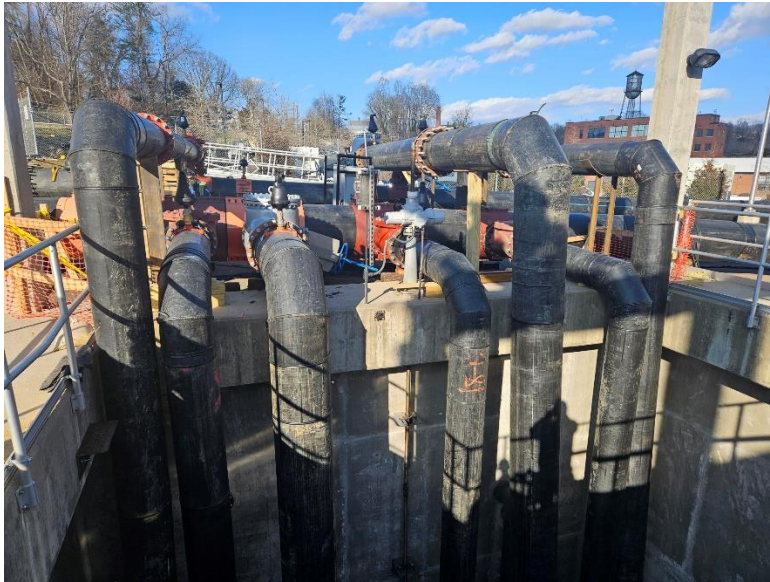
Bypass system pipes in the wet well
