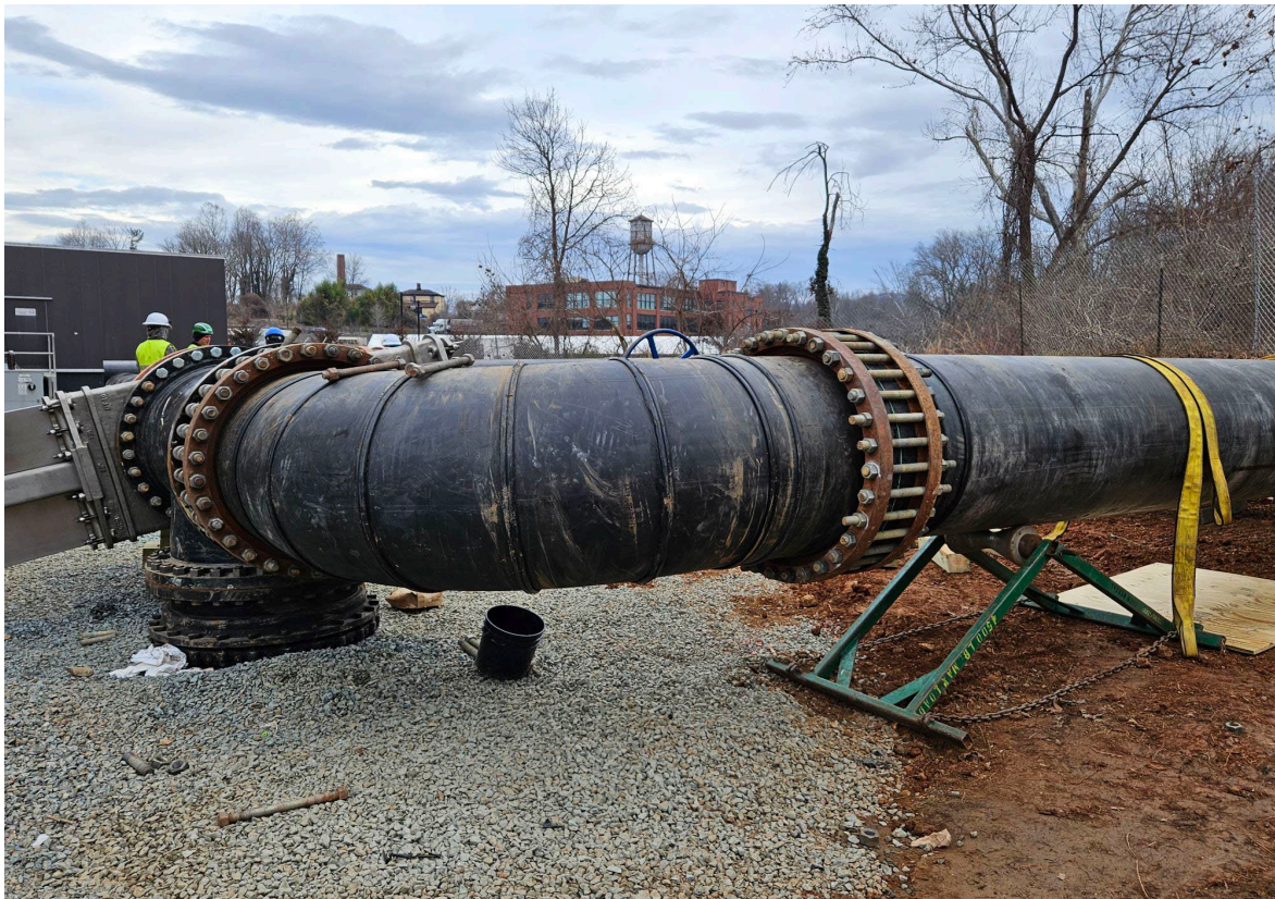
50 million gallons per day pumping bypass system
