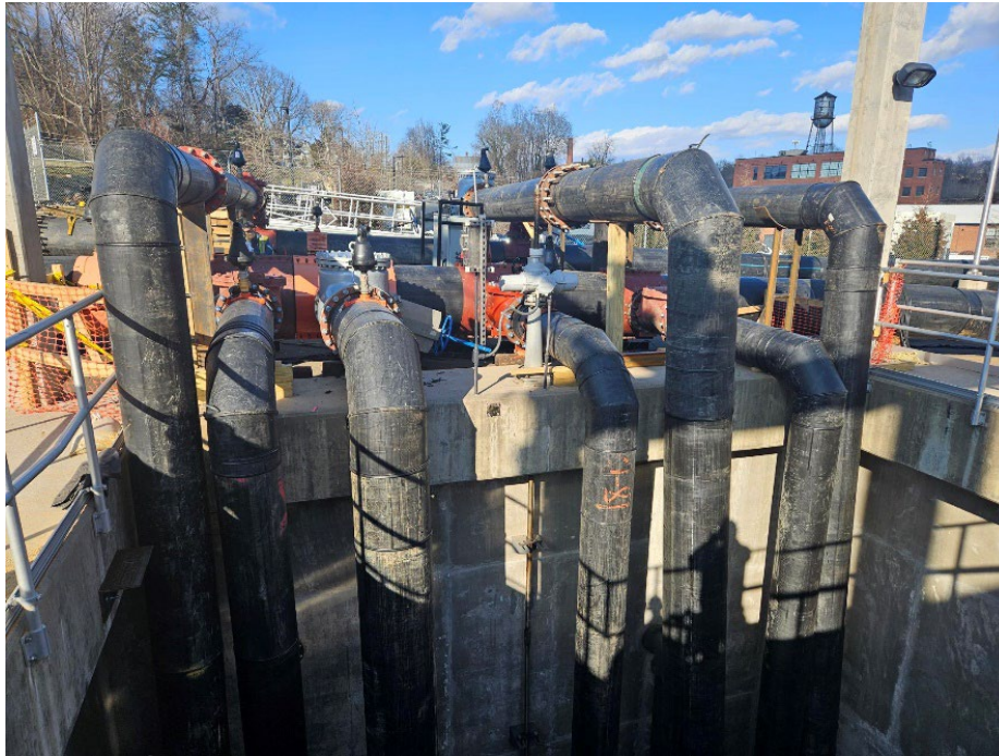
Bypass system pipes in the wet well.
