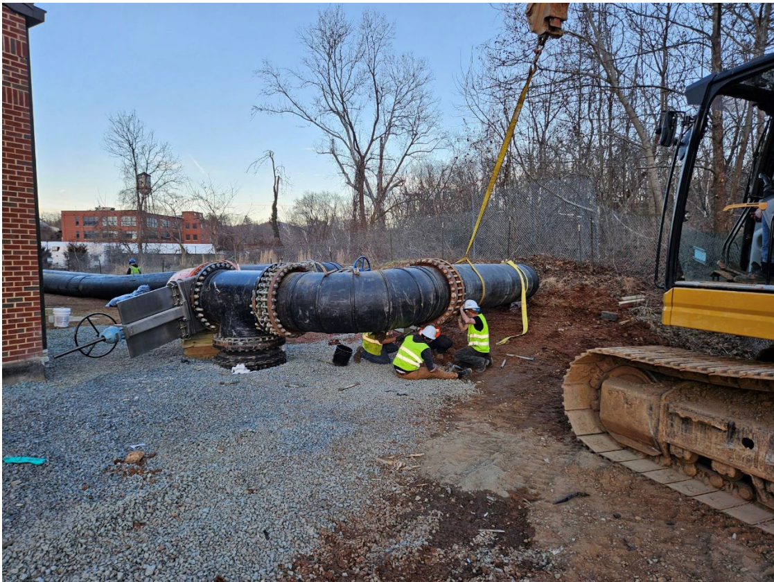
Bypass system pipes
