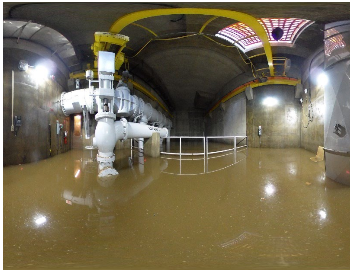
Submerged pump station pump room
