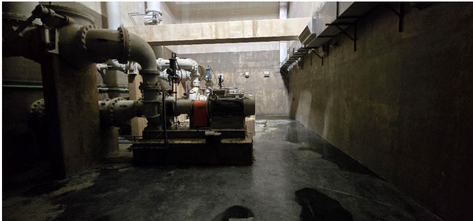
Cleaned pump room.
