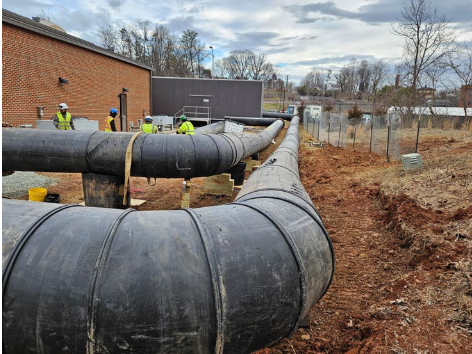
Large bypass system pipes
