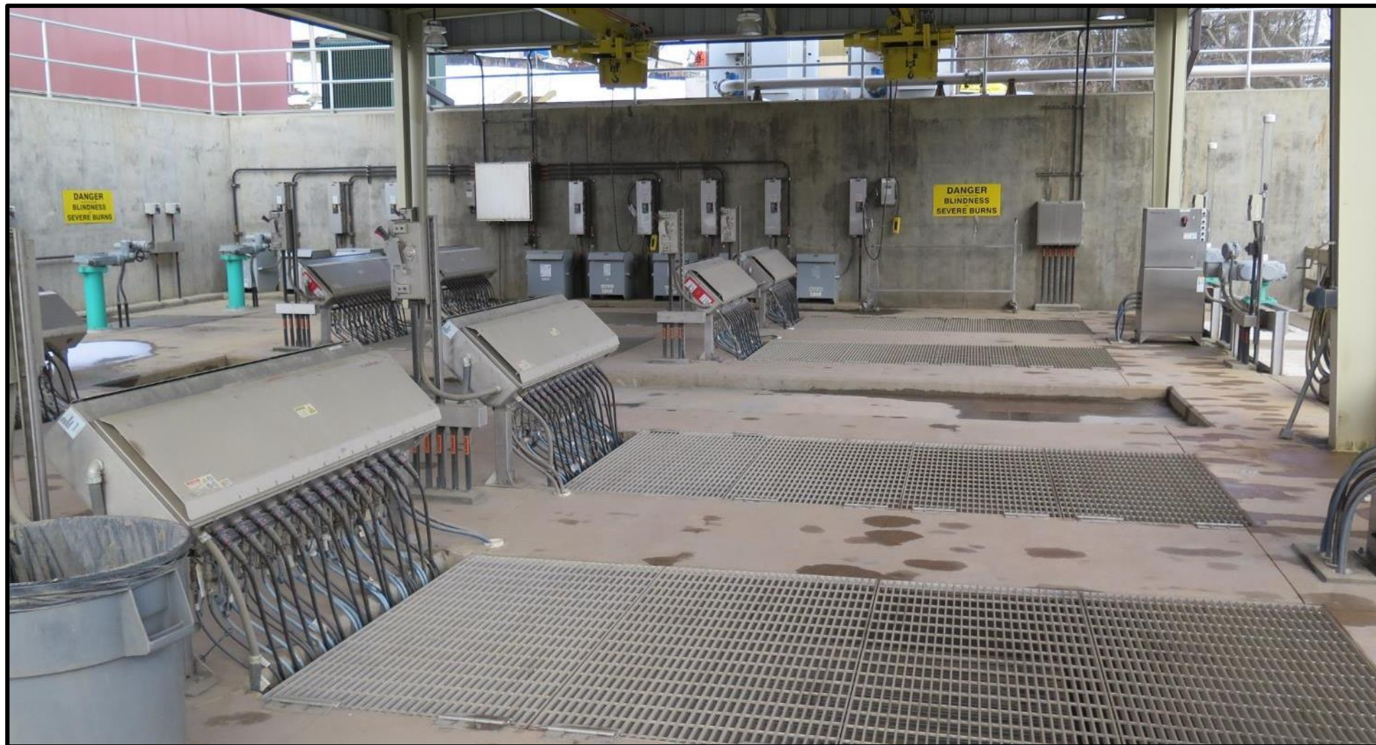
Ultraviolet light channels disinfects wastewater effluent flow
