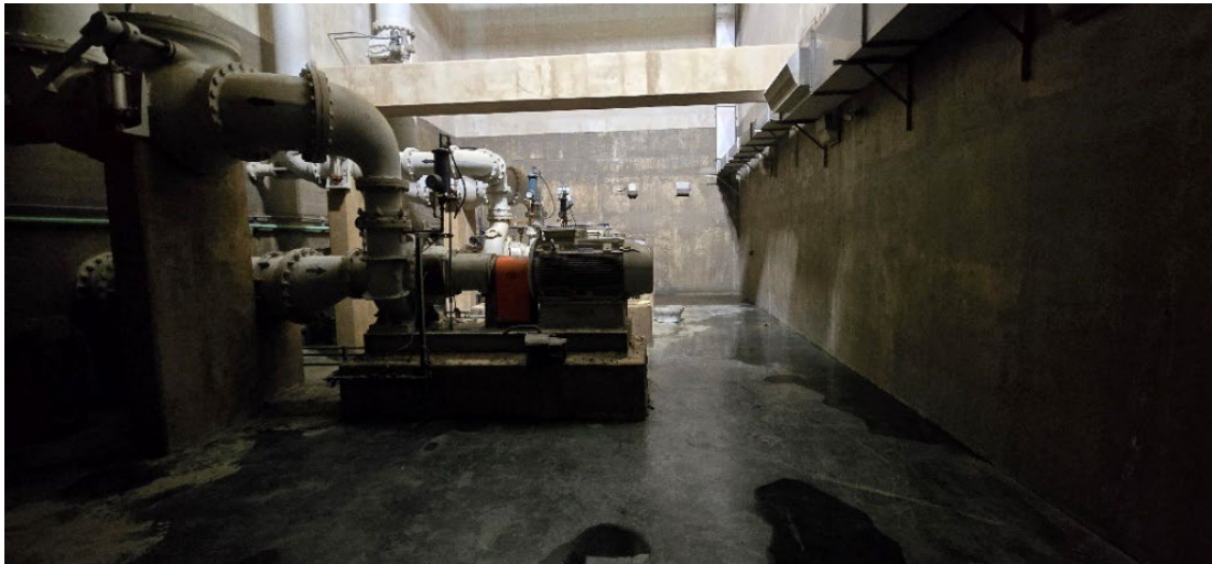
Cleaned pump room.
