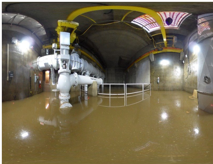
Submerged pump station pump room.
