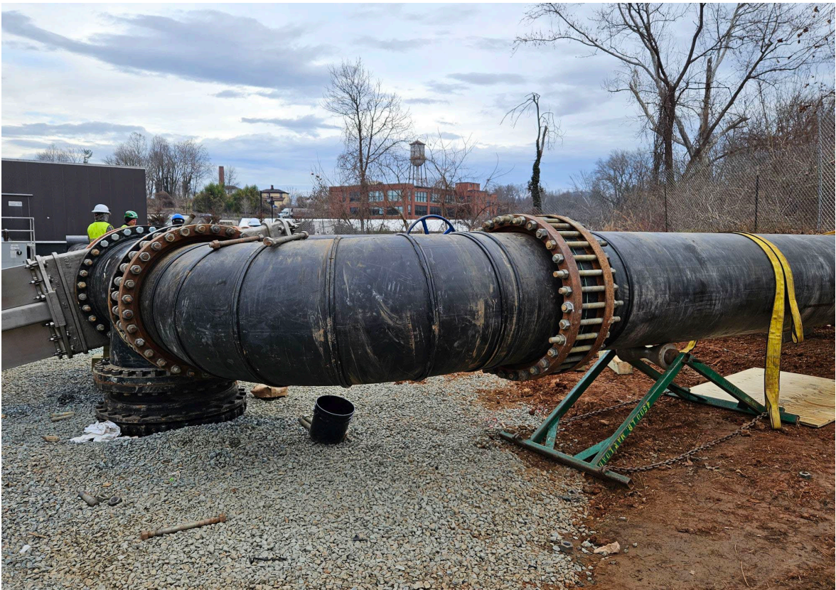
55 million gallons per day pumping bypass system
