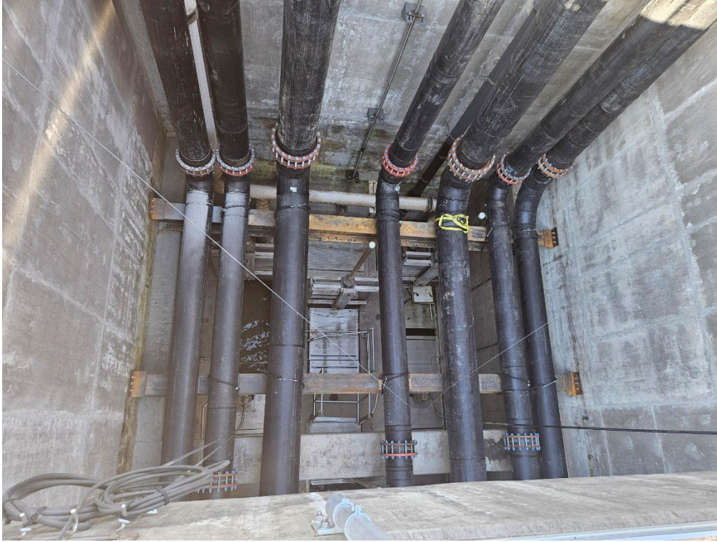
Bypass system pipes in the wet well.
