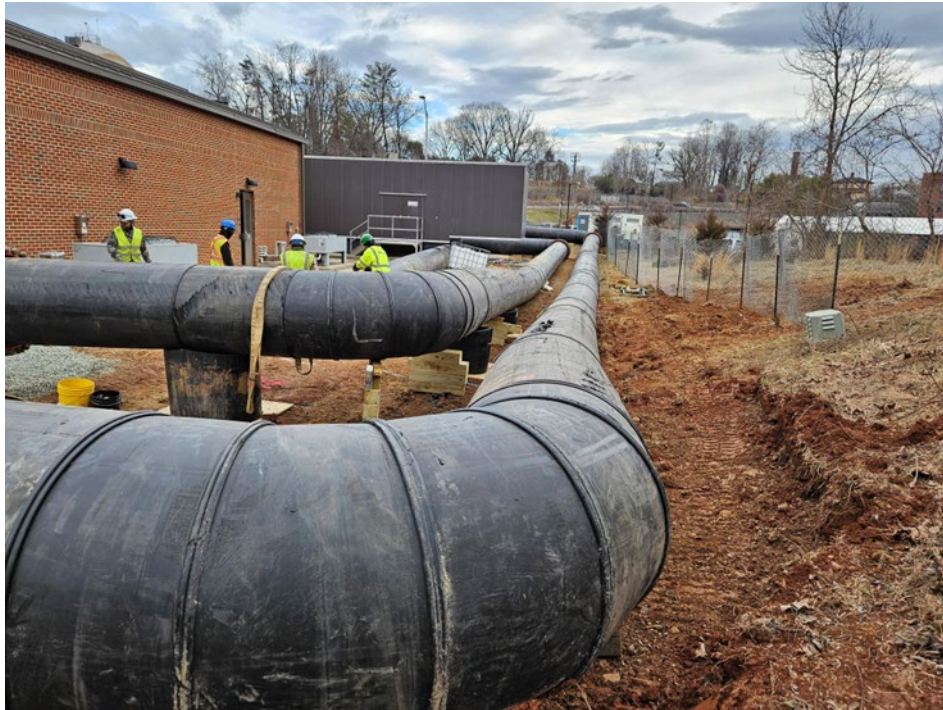
Large bypass system pipes
